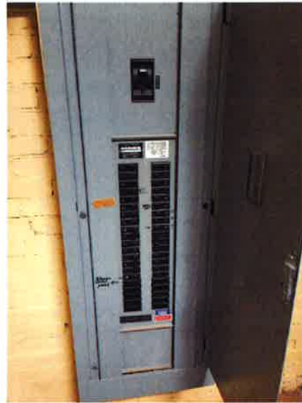
Typical basement electrical panel.
