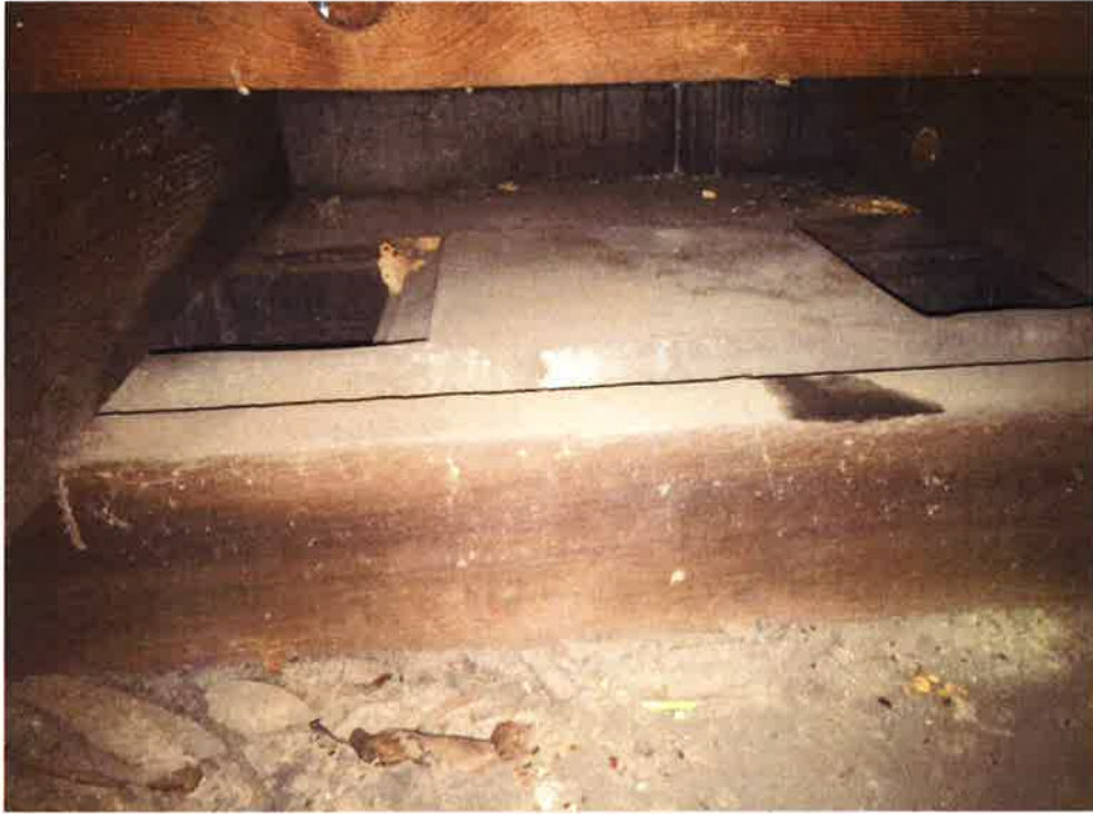
View of outrigger extension beneath exterior gutter. Note concealed top side of exterior decorative metal soffit.
