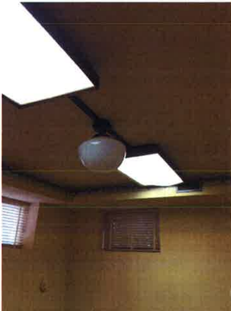
Basement – Typical room lighting
