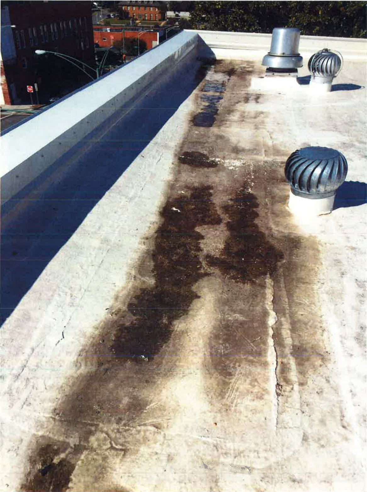
The flat roofs on the 1926 wings are holding water, specifically at the far south and far north edges.
