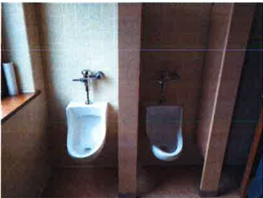
Typical wall mounted urinal with manual flush.
