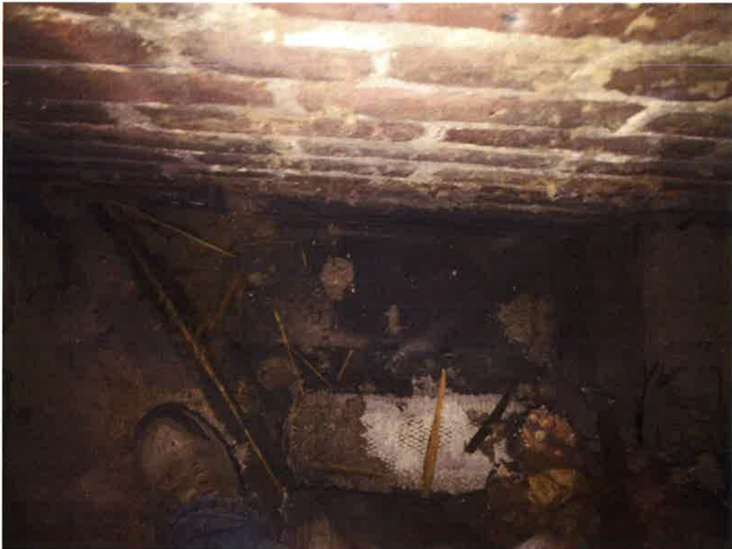
"Hip" beam bearing supporting courtroom ceiling. Note deterioration.
