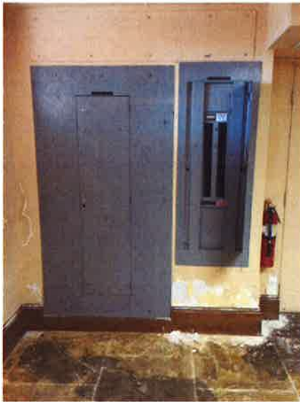
Basement – Flooding at main panel.
