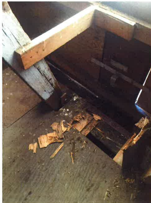
Isolated deterioration of clock tower framing.
