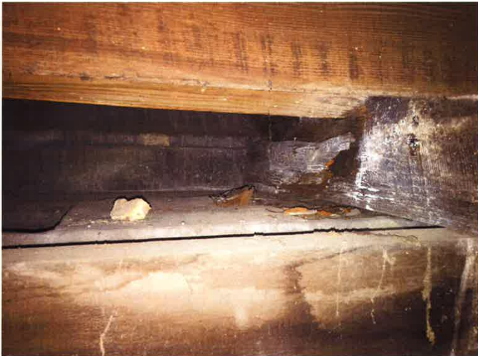
Crushed and deteriorated outrigger supporting roof purlin.
