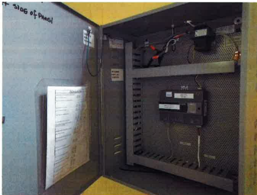
Basement – Johnson Controls building automation panel in utility room.
