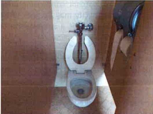
Typical wall mounted water closet with manual flush valve.
