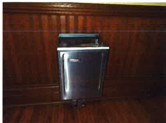
Typical single level water cooler.
