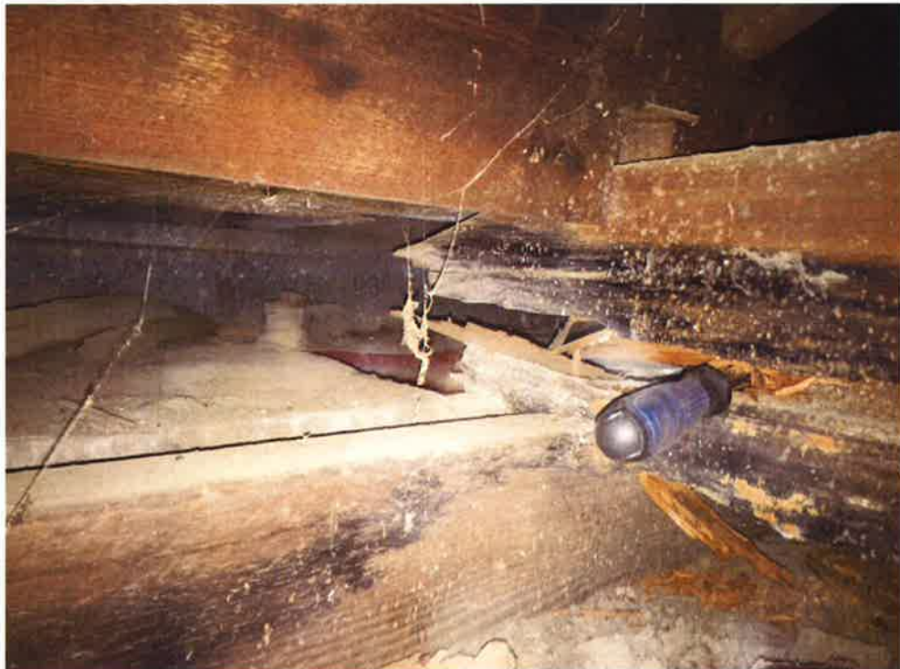
Deteriorated and crushed outrigger supporting gutter.
