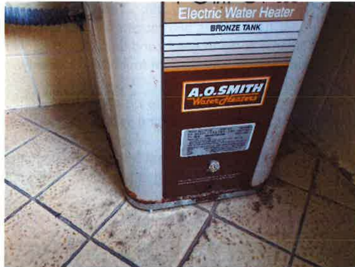
Instantaneous water heater beginning to rust at base of unit.
