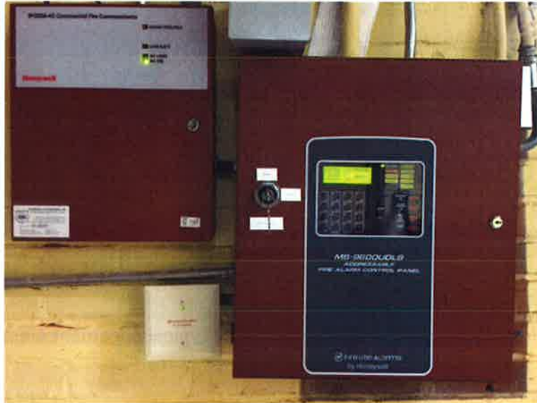
Basement – Existing Fire Alarm panel.
