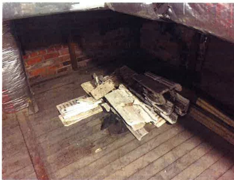
Unused fiber-reinforced (blue plastic mesh) plaster units from 1990s plaster work.
