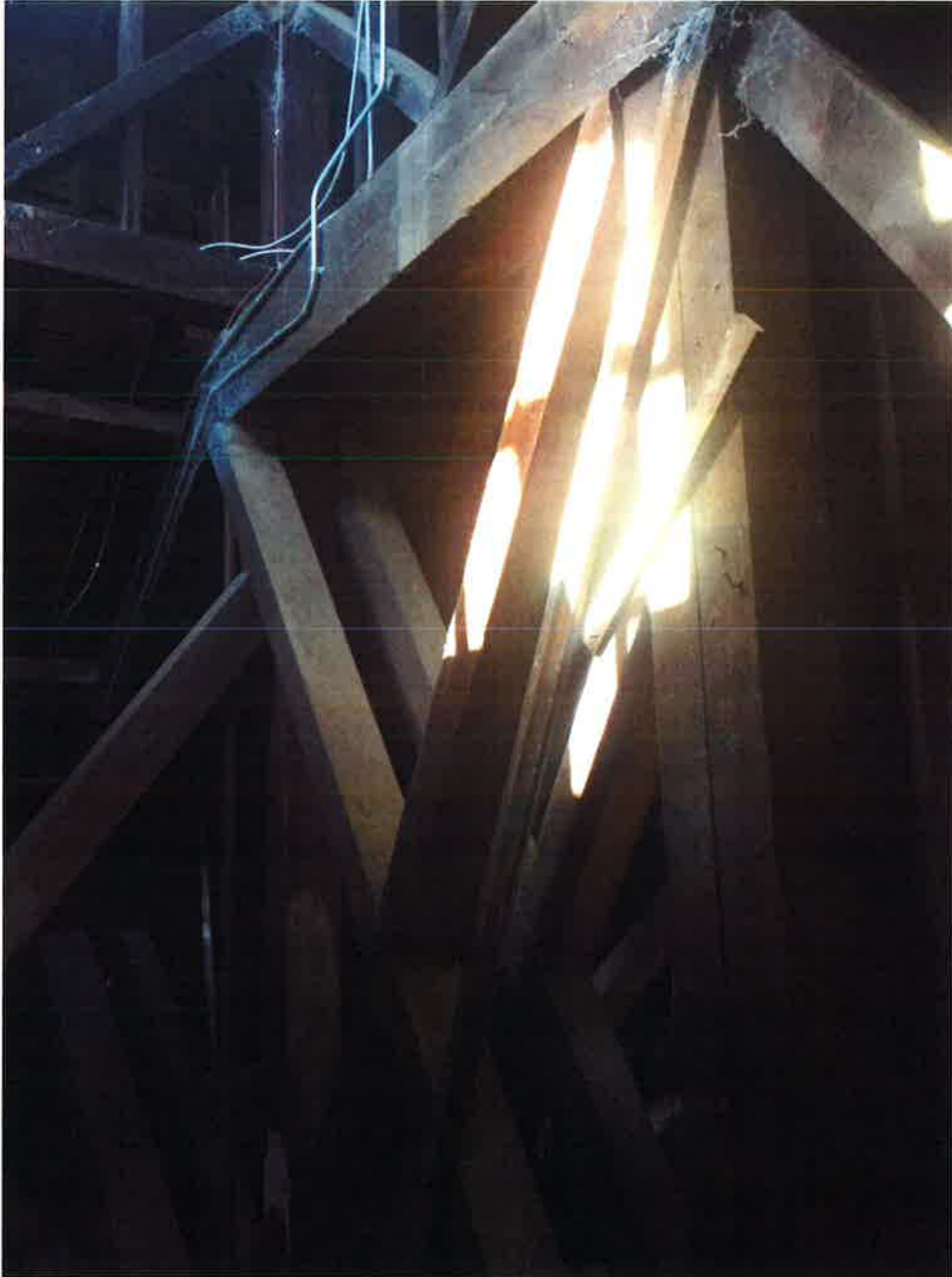
Diagonal web members of main roof trusses. In some cases these diagonal web members are loose.
