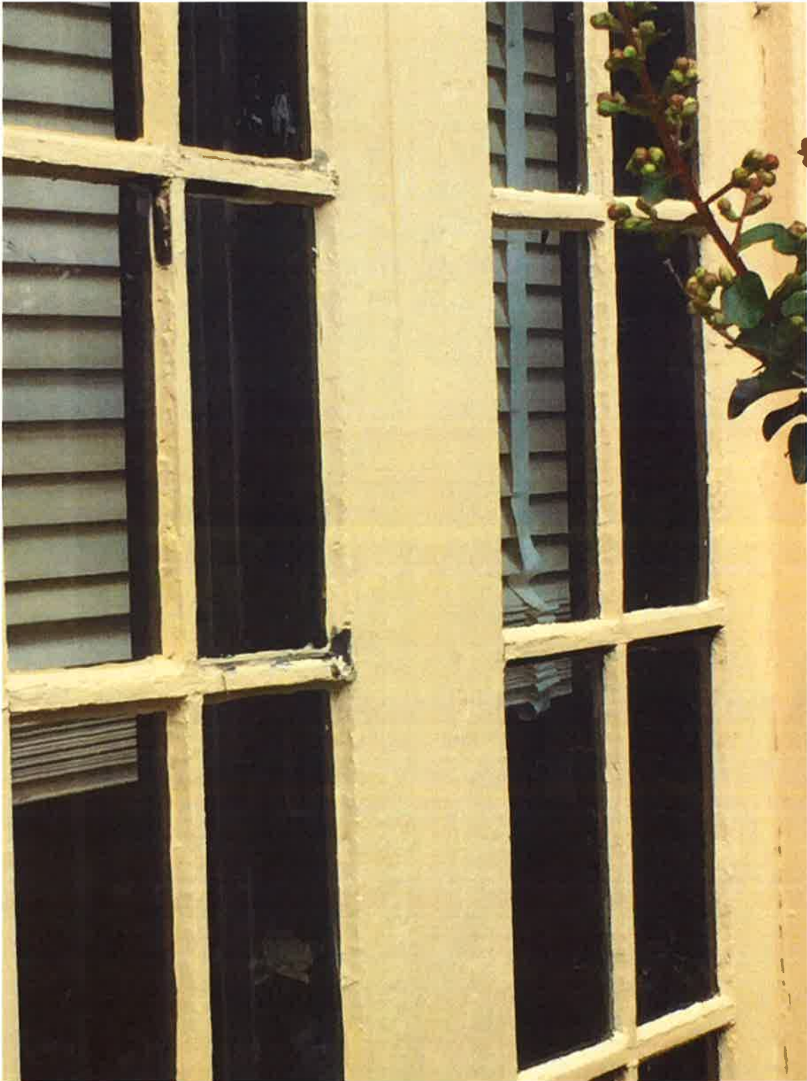
Exterior window muntins appear to have been rebuilt with wood filler and hastily re-glazed in several locations.
