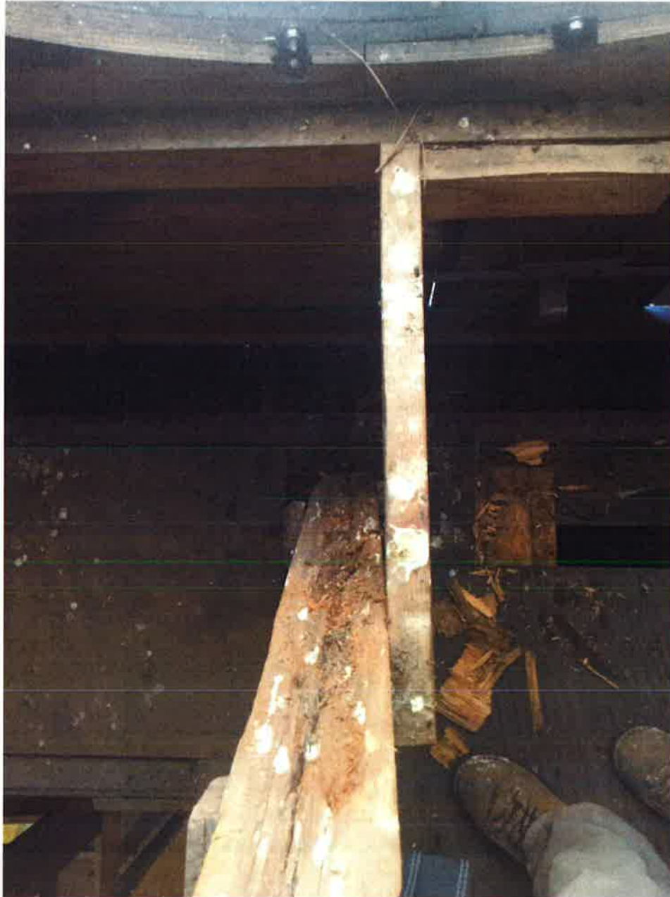
Isolated deterioration of clock tower framing.
