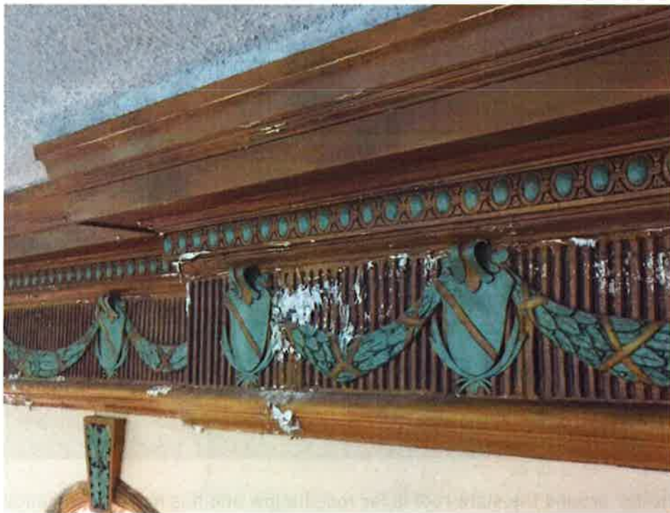
Water penetration from the slate roof and box gutter, has caused significant deterioration of the plaster frieze in the courtroom below.
