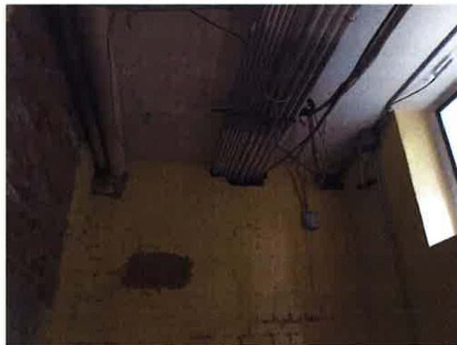
Basement – Conduit penetrations not fire-sealed.
