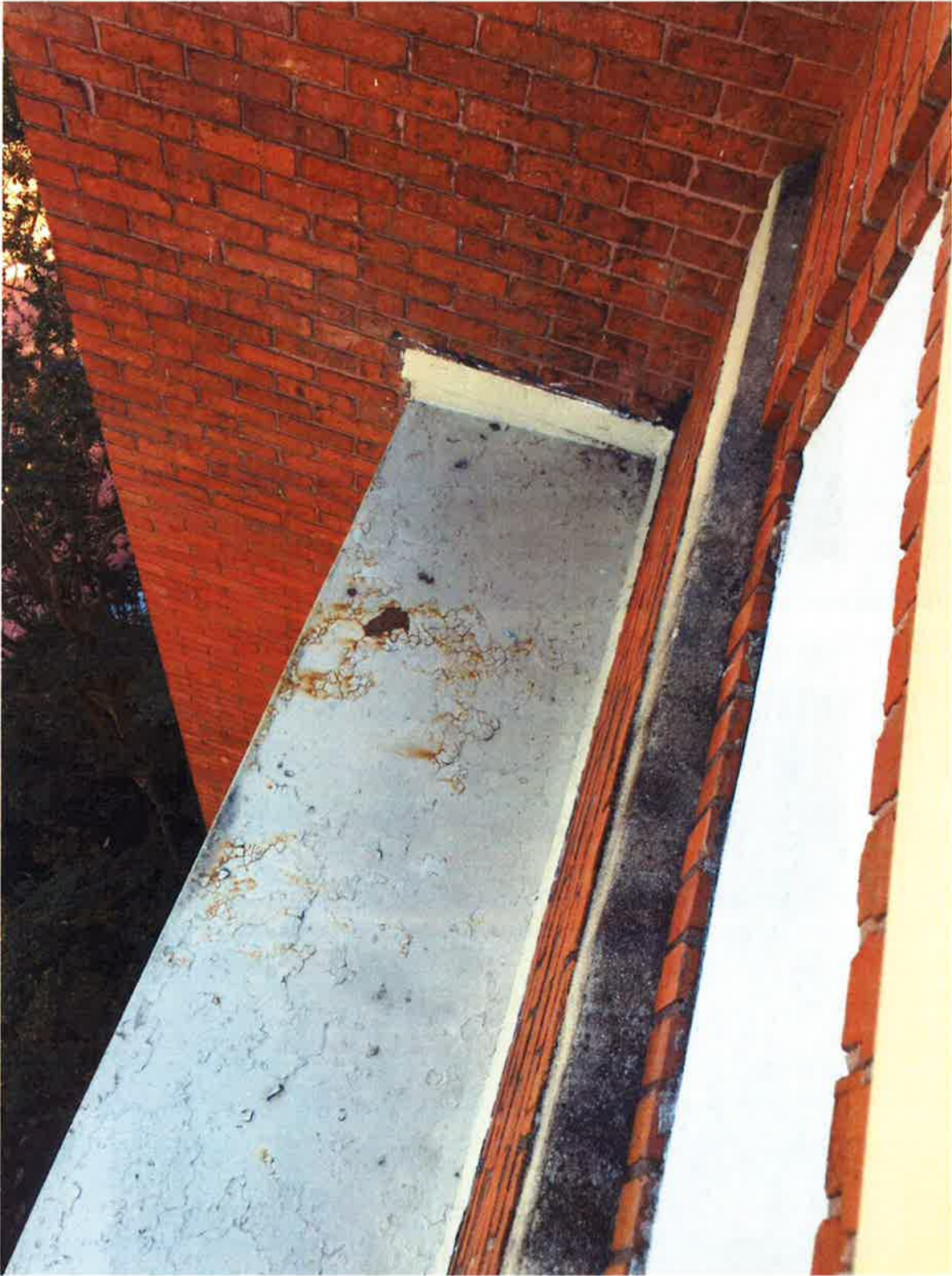
The pent eaves at the 1926 wings are beginning to spot rust in many areas.
