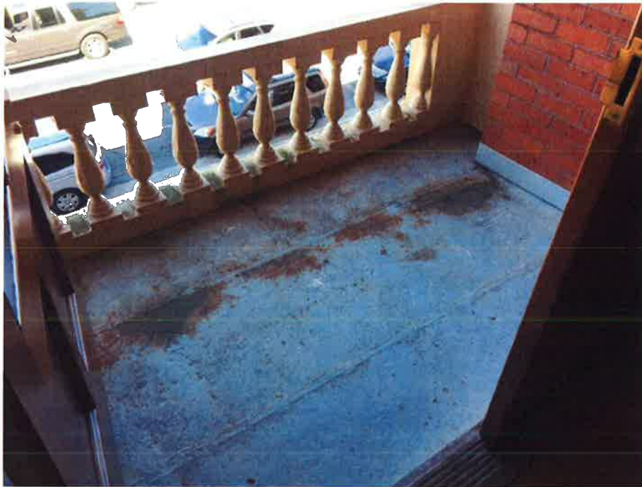
The flat seam metal at the balcony flooring has begun to corrode.
