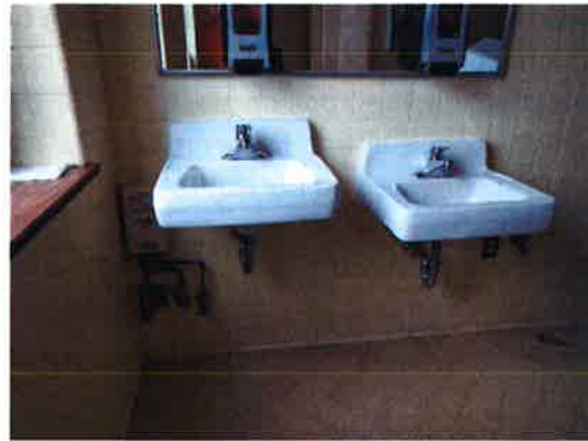
Wall mounted lavatories and instantaneous water heater serving two gang toilets.
