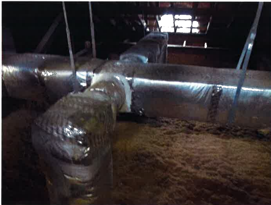
Supply duct in attic.
