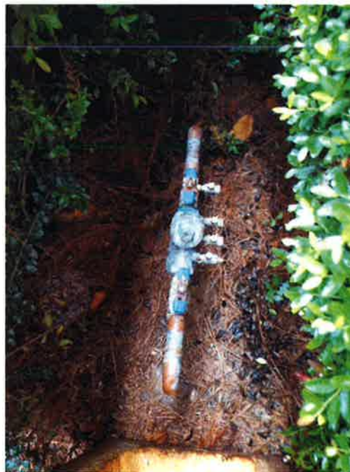
Domestic water backflow preventer adjacent to crawlspace.
