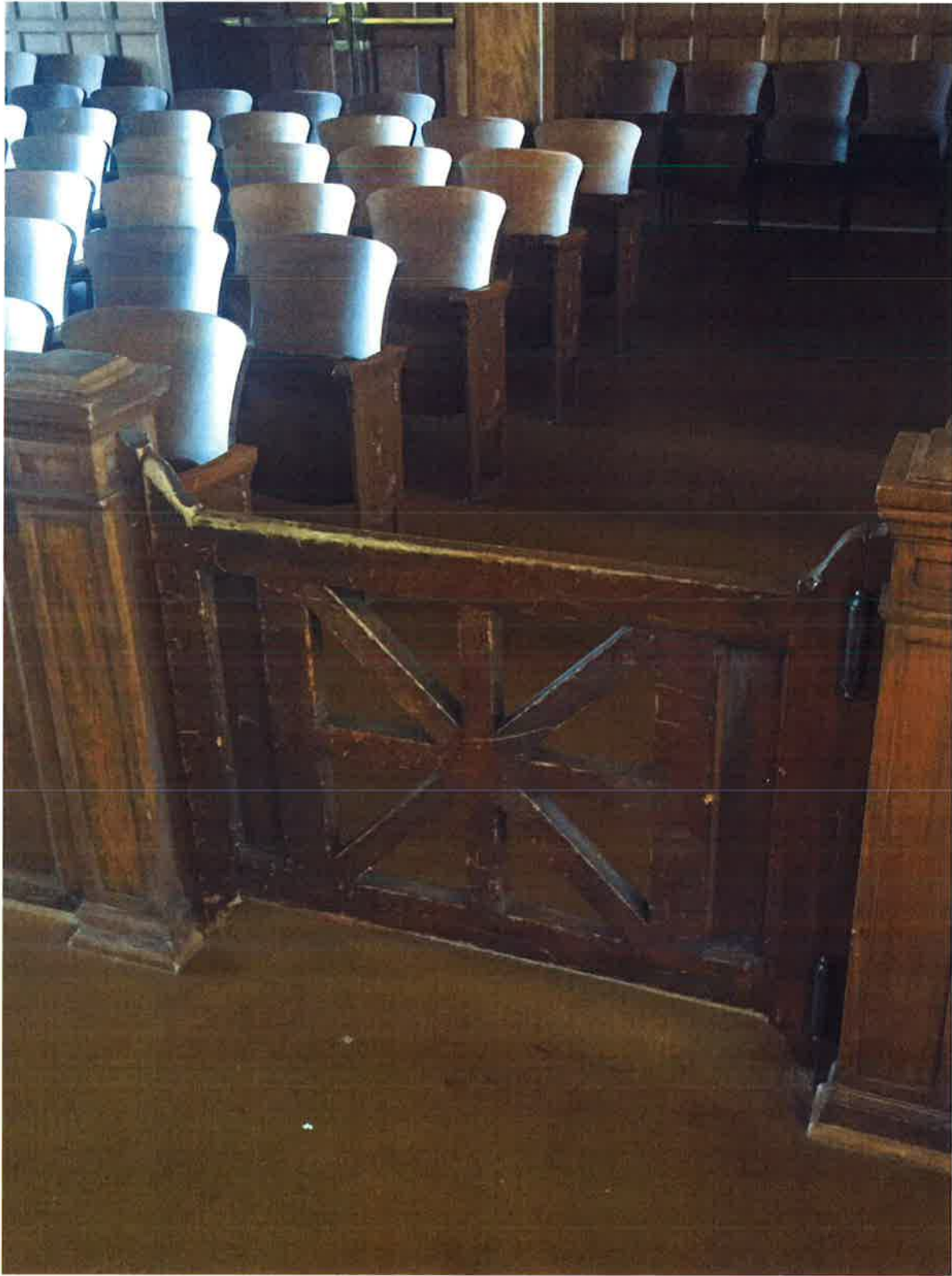
The finish on the top rail of the gates at the courtroom bar is worn away from use.
