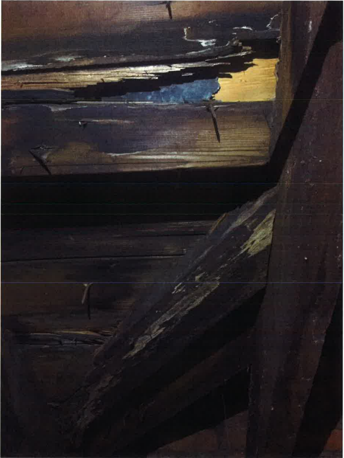
Deteriorated framing at gutter.
