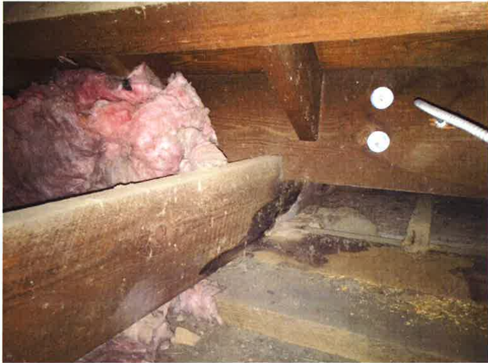
Deteriorated outrigger extension supporting roof framing.
