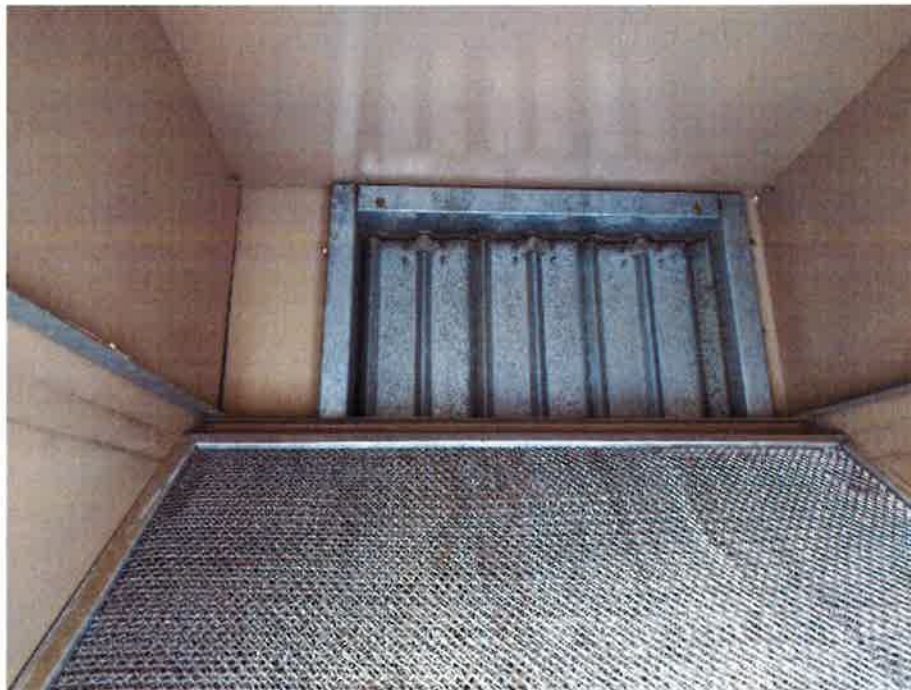
DX air handling unit outside air damper closed.
