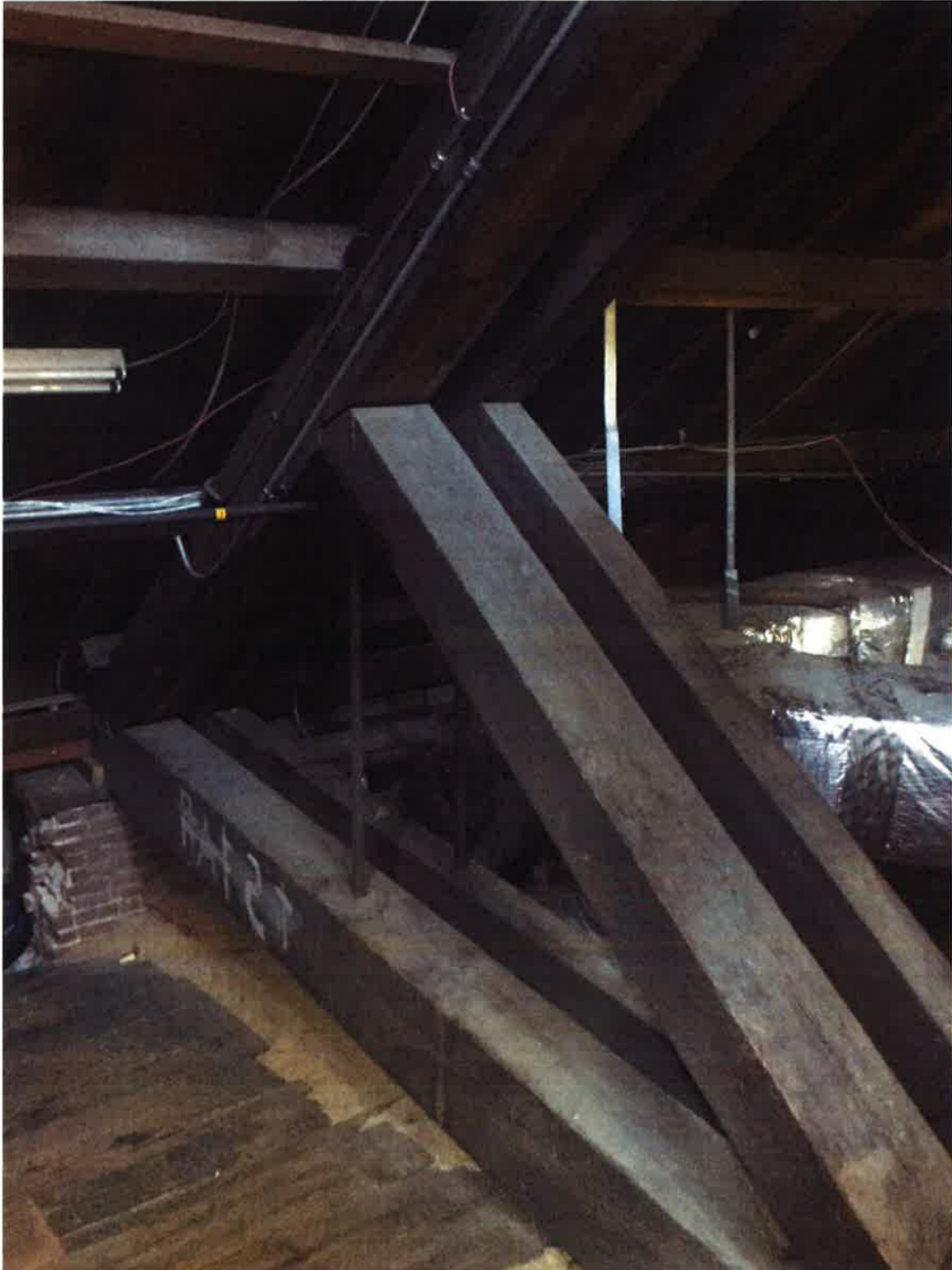
Roof truss web members. Note gap between timber web and chords. Integrity of connection depends on bolt tension on connection.
