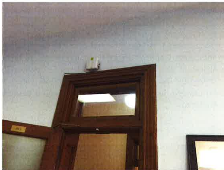
First Floor - Wireless access point.
