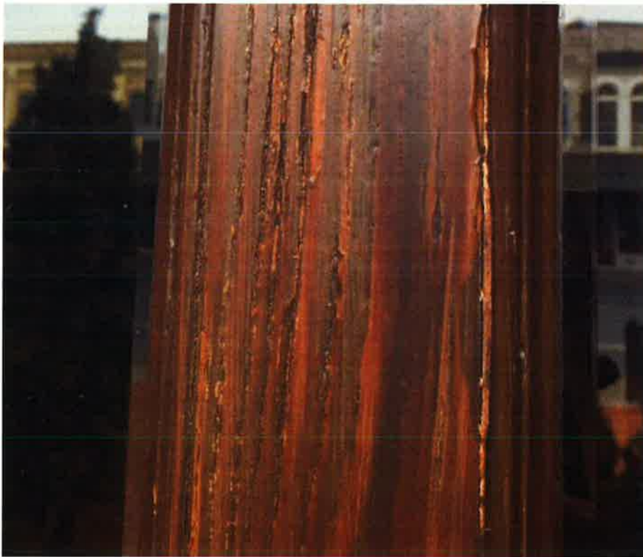
The finish on the exterior doors, specifically the south pair of doors, has begun to fail.
