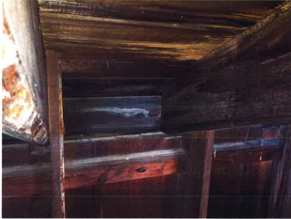
Water penetration at the slate roof can be seen as water staining and damage to the roof plate, rafters and decking below.
