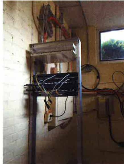
Basement - Telephone service.
