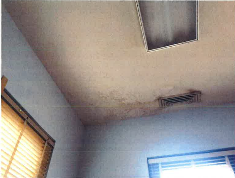
Water has damaged the ceiling in the room at the NW corner of the second floor.
