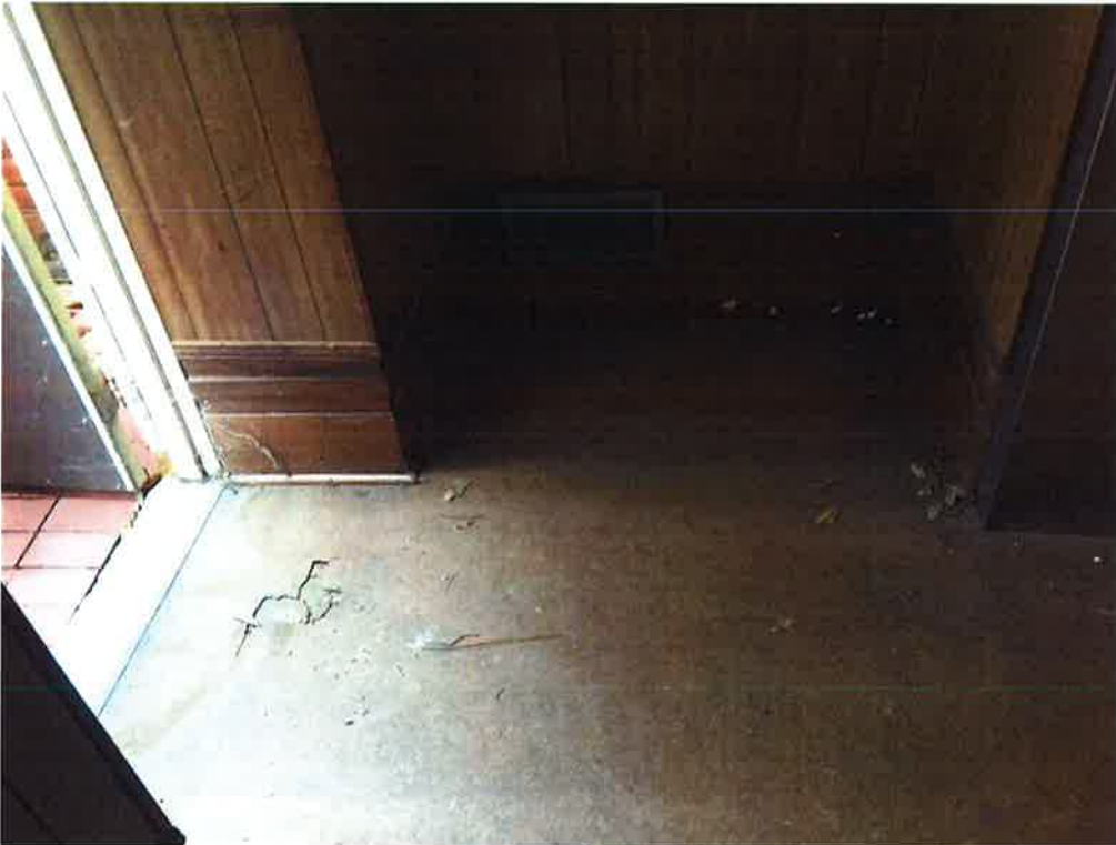
Water penetration at the handicap ramp into the elevator lobby appears to be due to a clogged drain at the base of the ramp.
