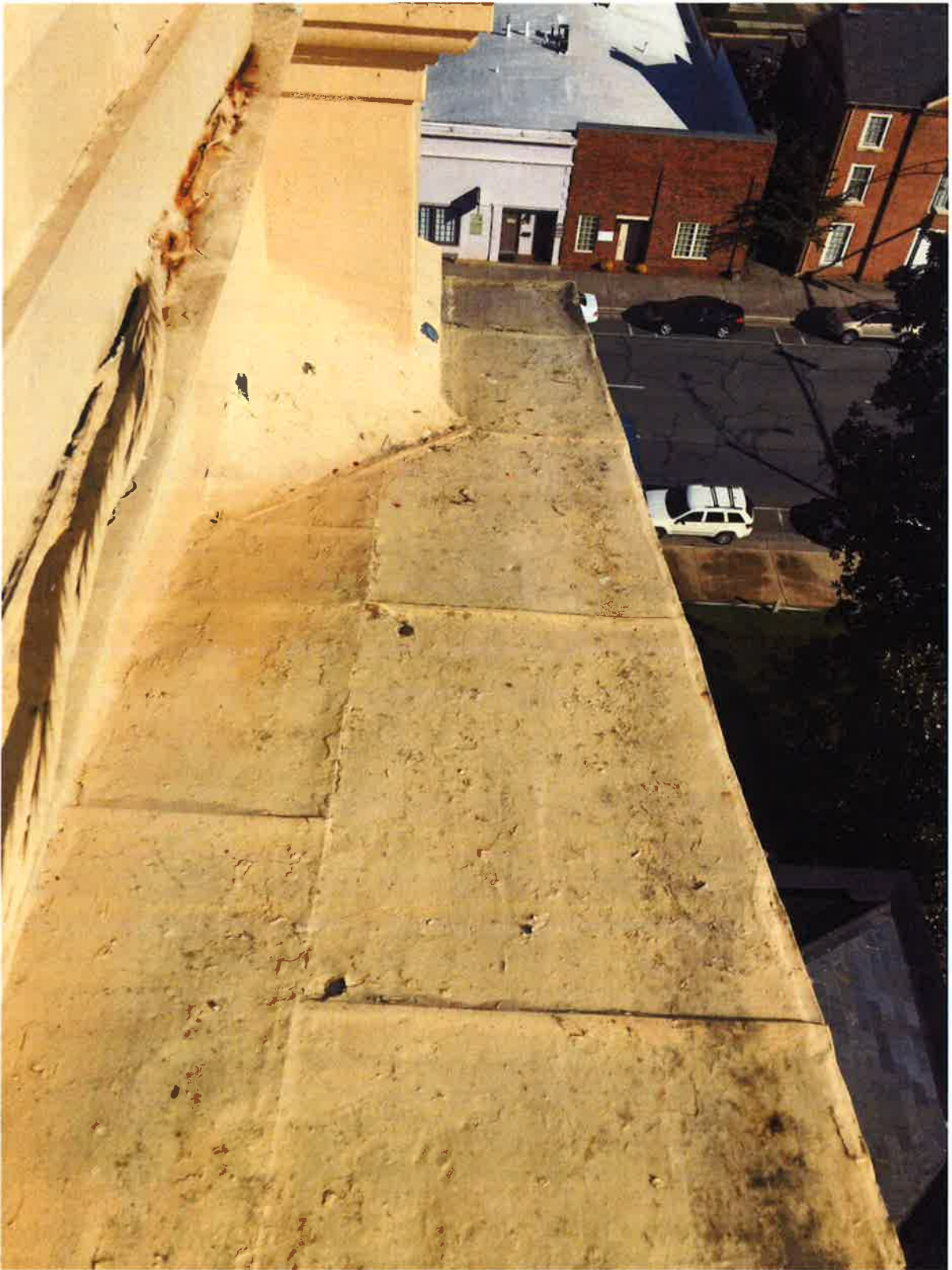
The sheet metal roofing just below the clocks is in good shape, with only minor areas of rust and paint loss.
