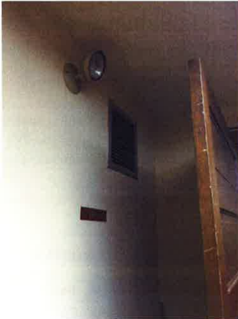
Basement - Egress light is blocked by door.
