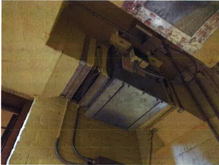
Basement – Exhaust fan installed in utility room.
