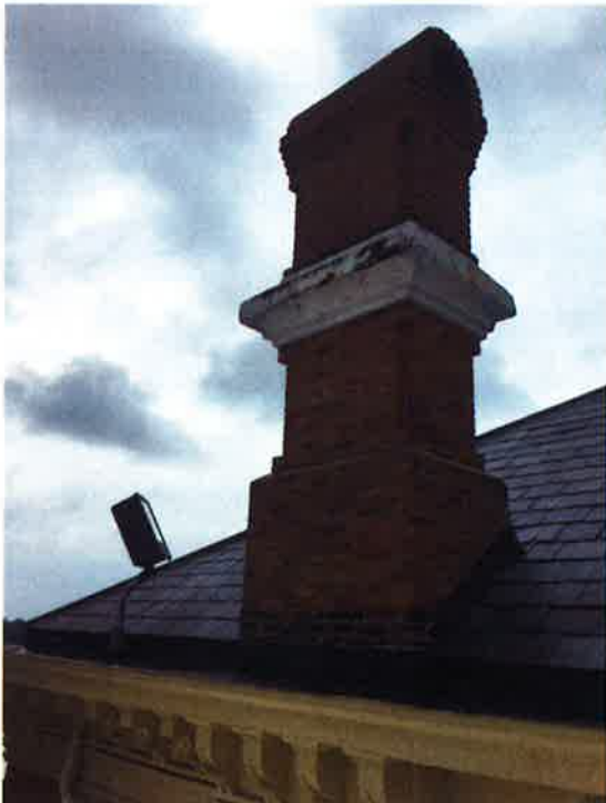
Roof – clock tower floodlight
