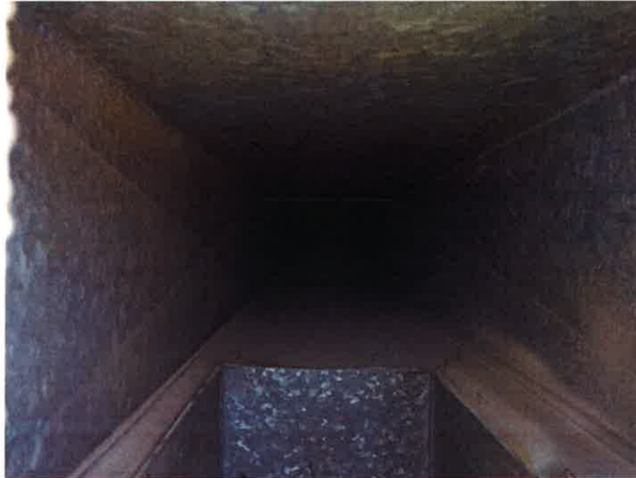
Inside of ductwork in attic. No significant accumulation of dust.
