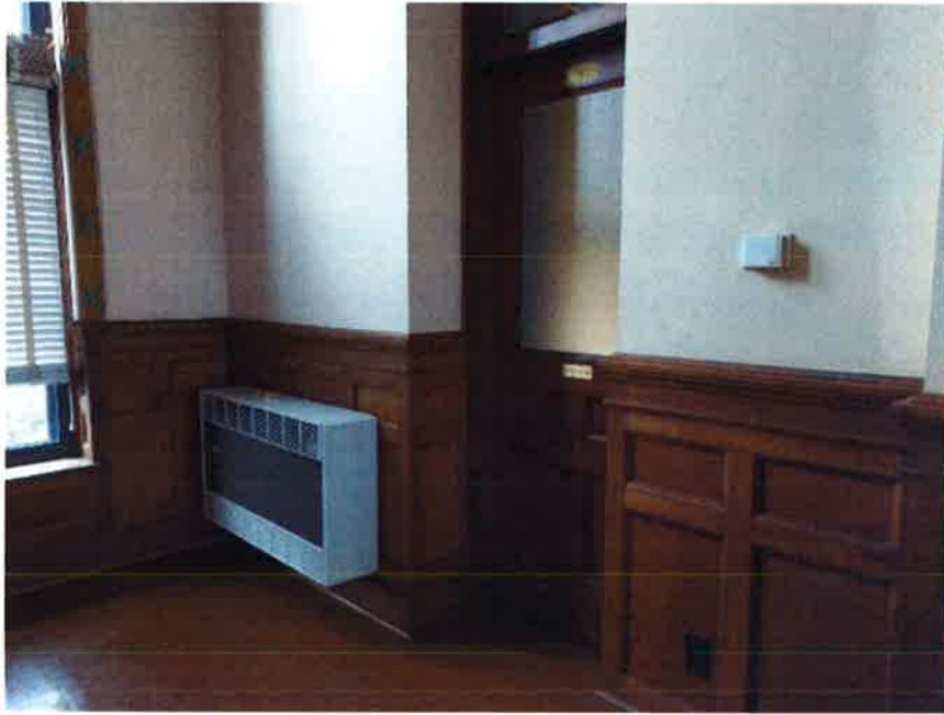
Second Floor – Electric heater in courtroom.
