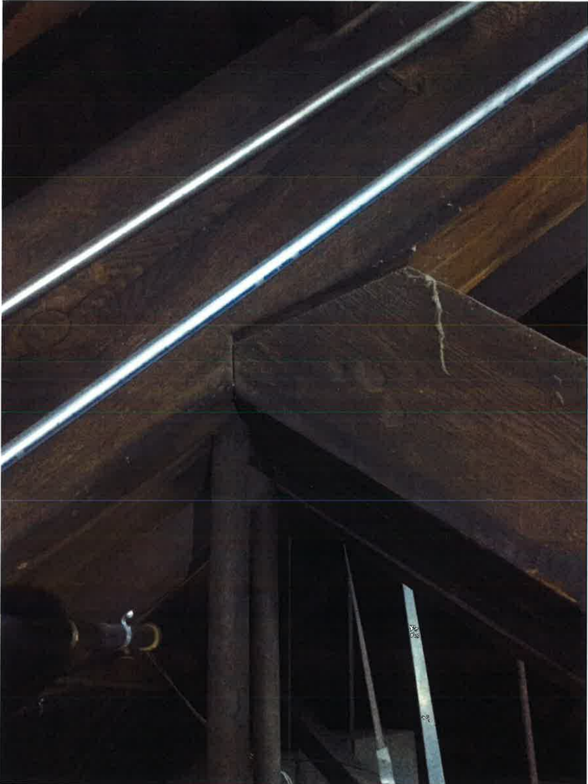
Loosened roof truss connection.
