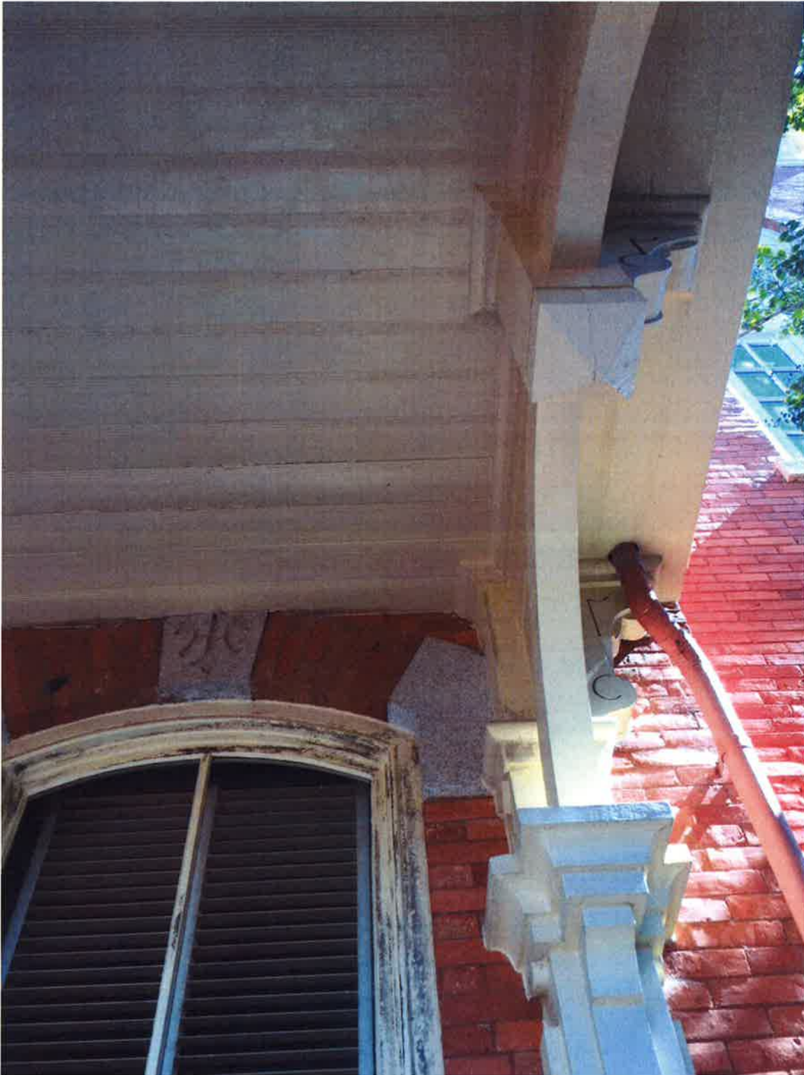
Moisture penetration from the roof above has caused paint deterioration at the portico ceilings and mildew at the windows.
