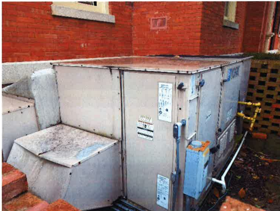
DX Air handling unit on grade behind screen wall.
