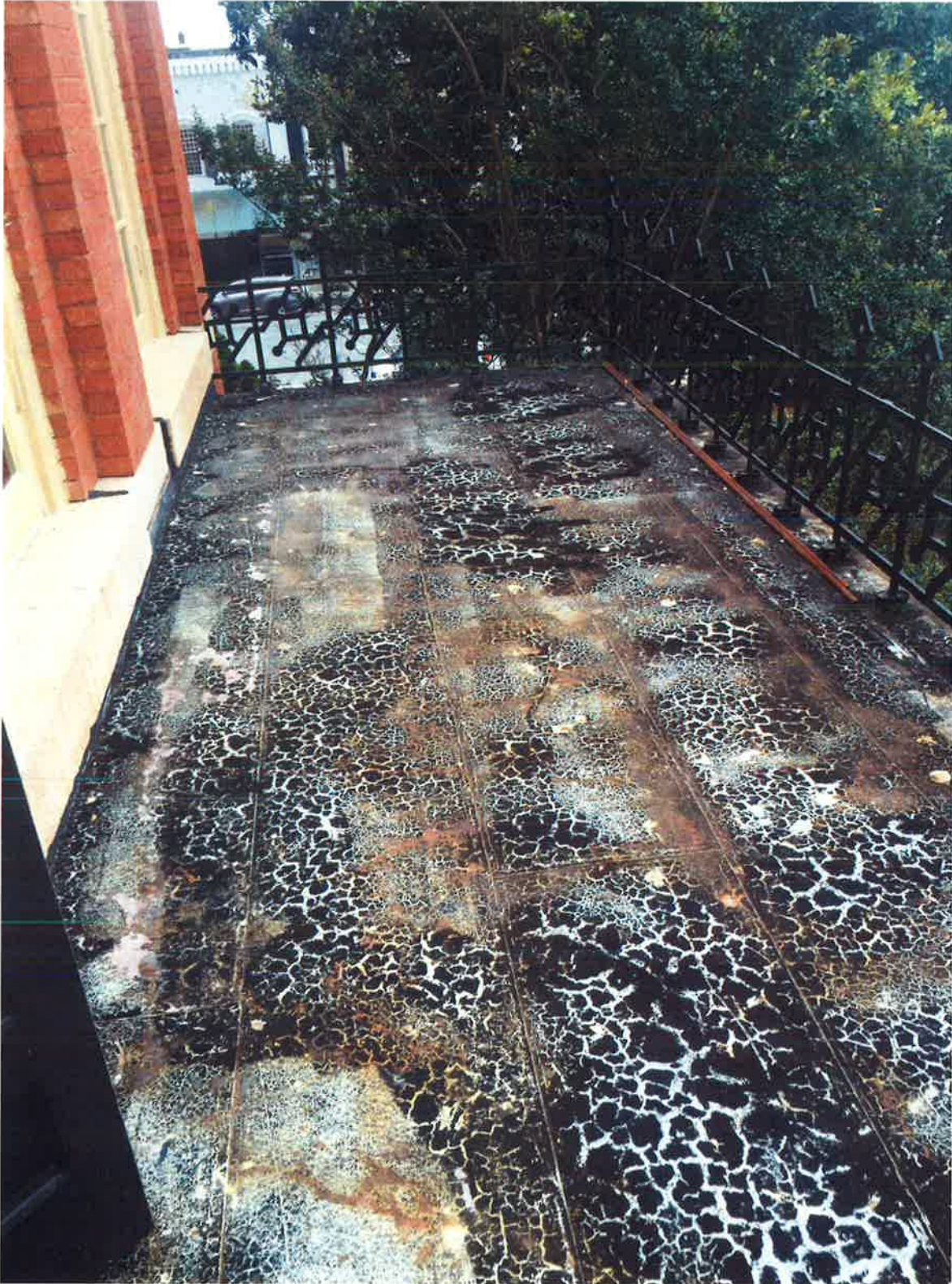
The flat seam metal roofing on the porticos has been covered with roofing tar which has crazed and eroded.
