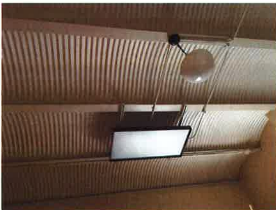
First Floor – Ligting in vault. Surface-mounted conduits.
