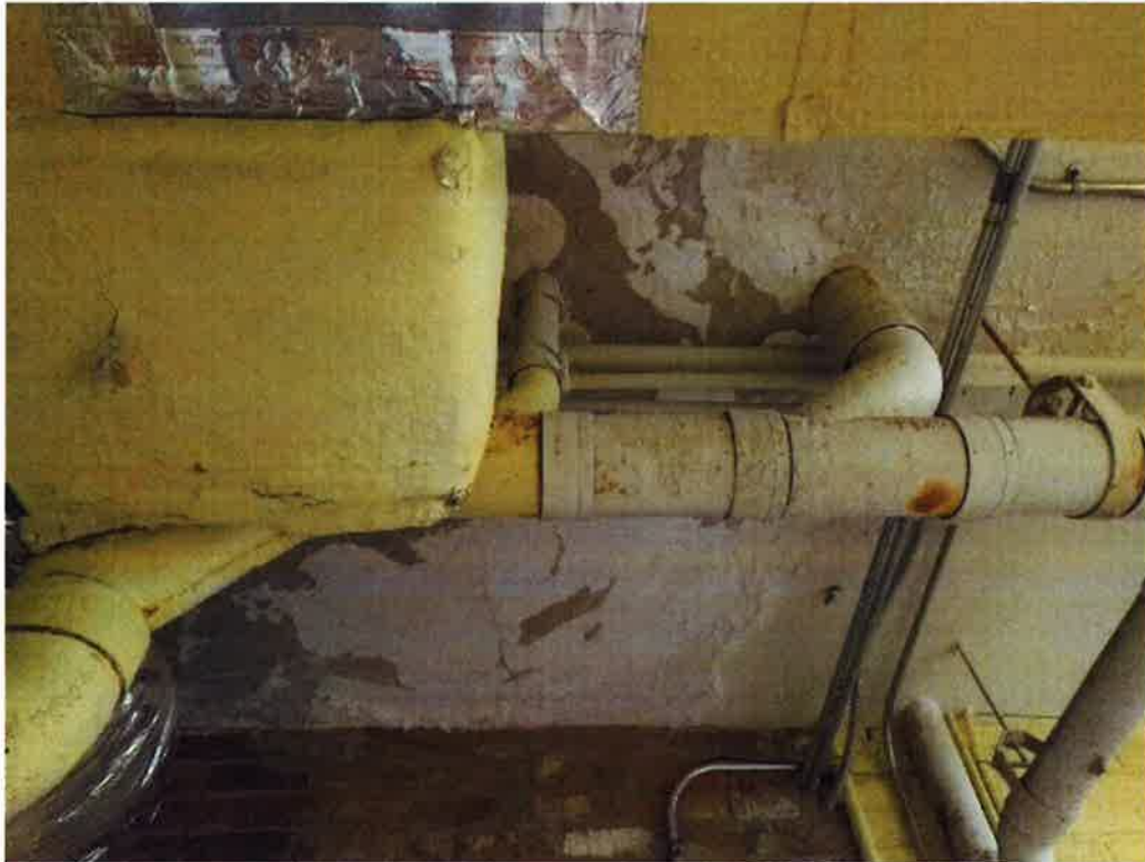
Basement – Cast iron waste pipe.
