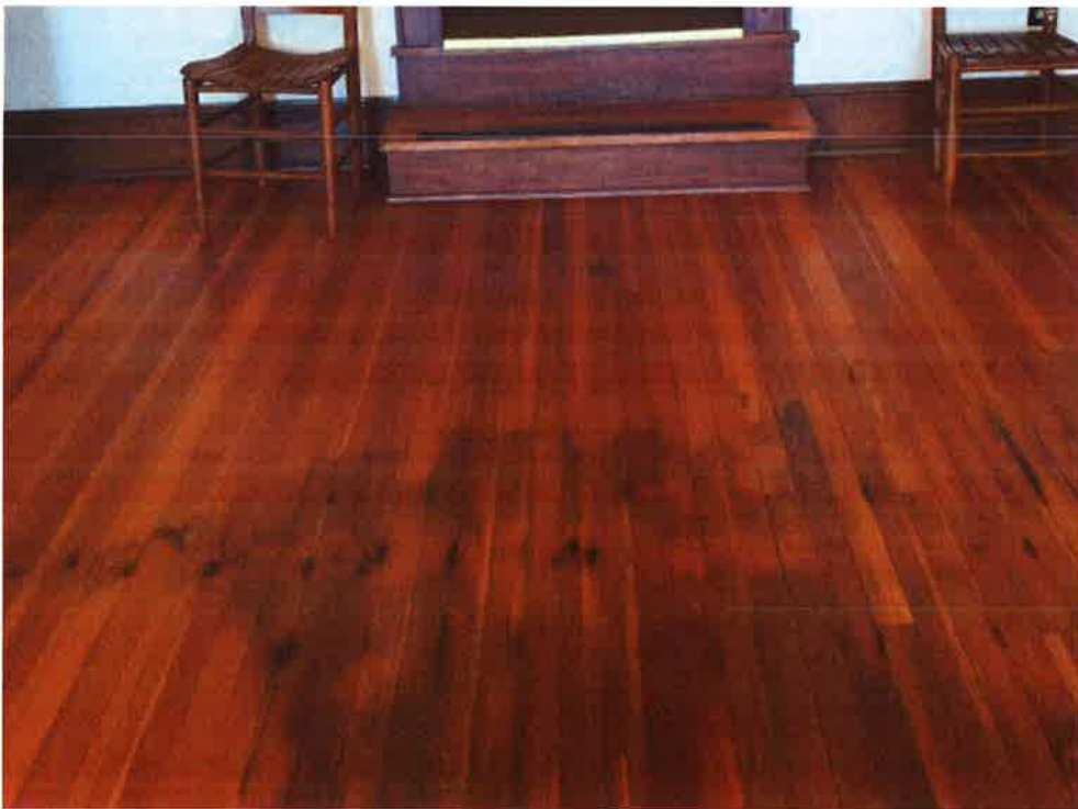
Past roof damage has caused water staining to the flooring in the room at the SE corner of the second floor.
