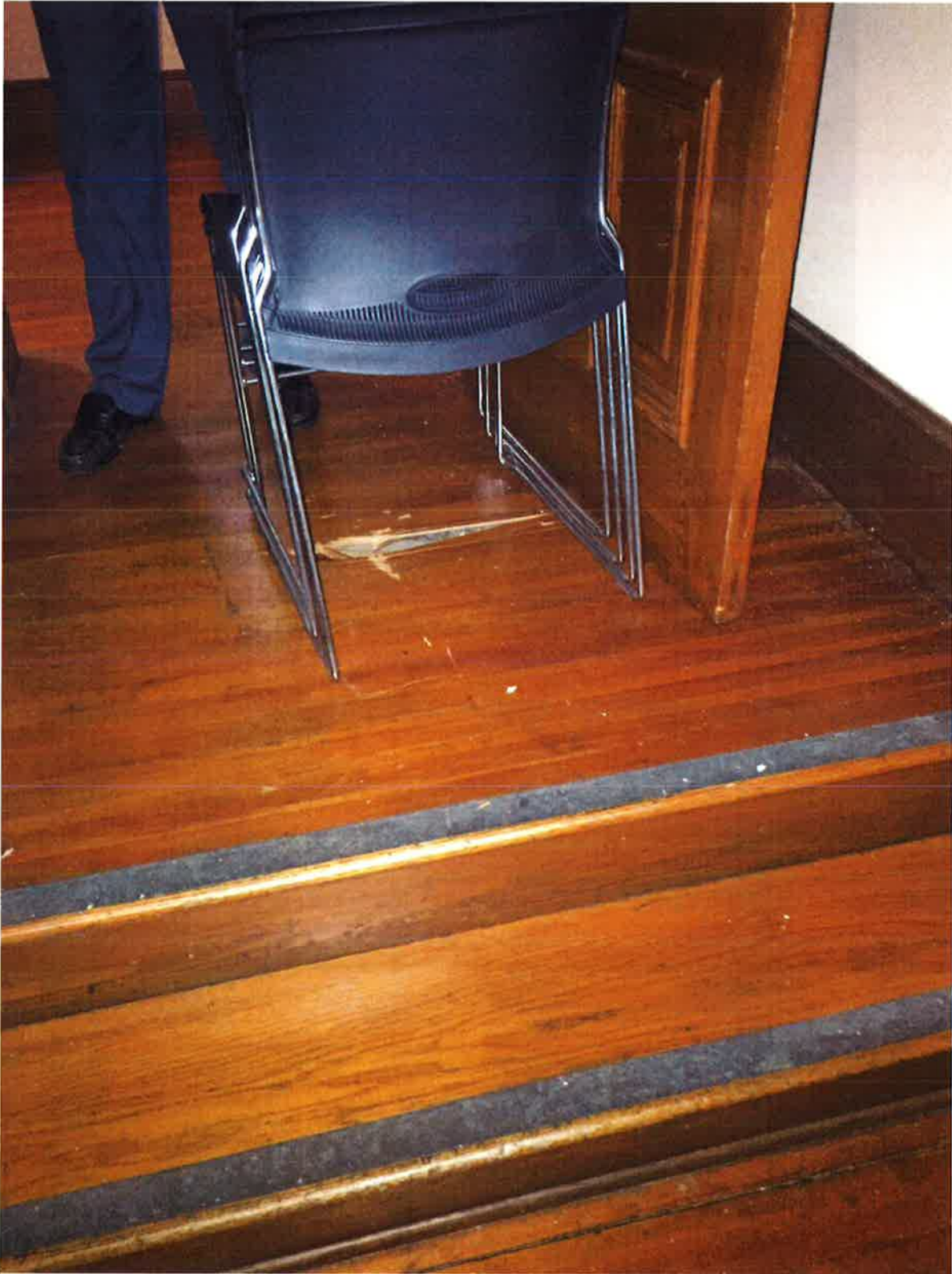
Flooring in the north stair hall was damaged by a past film crew.
